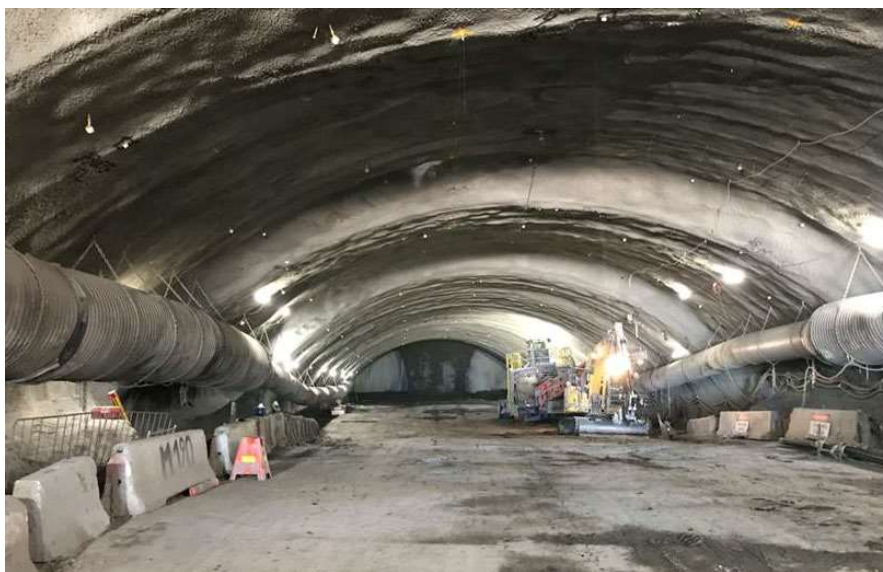
FIG 12 – Completed top heading for section with canopy tubes, steel sets and Bullflex system.
